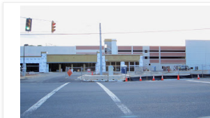
The shopping center on Annandale Road being developed by Bill Page Honda.
